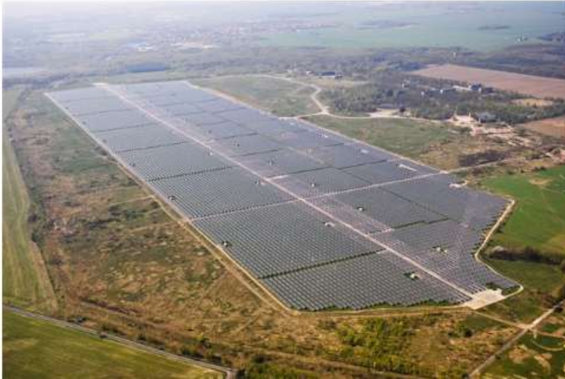
PV as large as airports (Saxony, Germany)
