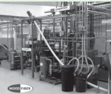
Compounding plant for the production of WPC Wood Plastic Composites.
