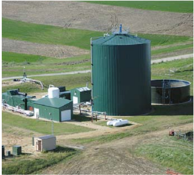
Wild Rose manure digester facility in Wisconsin, Dairyland Power Cooperative
